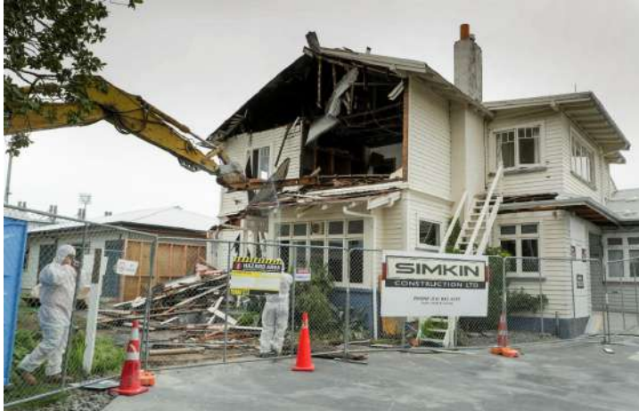
Demolition of 42 Morris Street by Simkin Construction. Note men in safety gear because of asbestos in building. Photo / Warren Buckland, 2020
